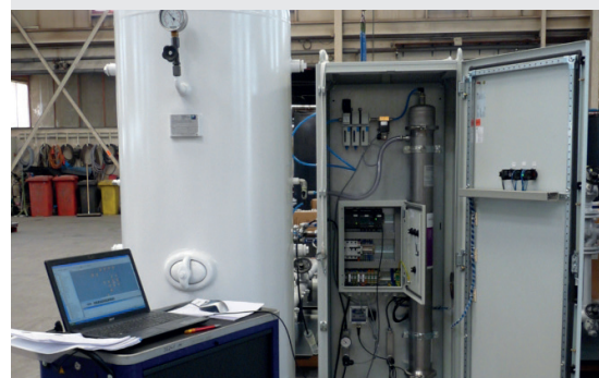
Open Nitrogen Generator
