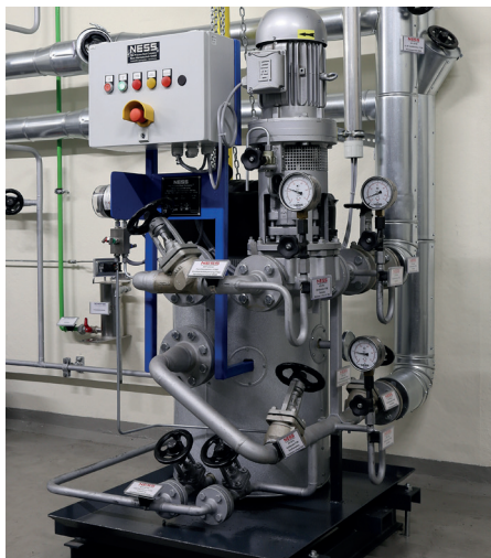
FF300 integrated in plant
